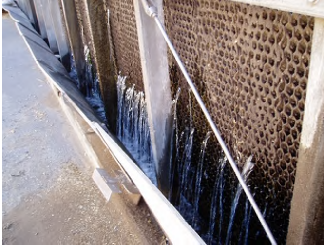
Plugged fill and heavy scale.
