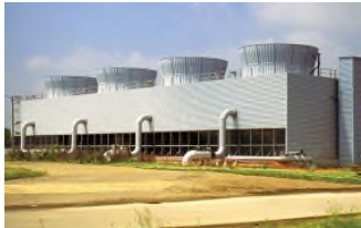
Marley Industrial counterflow tower
